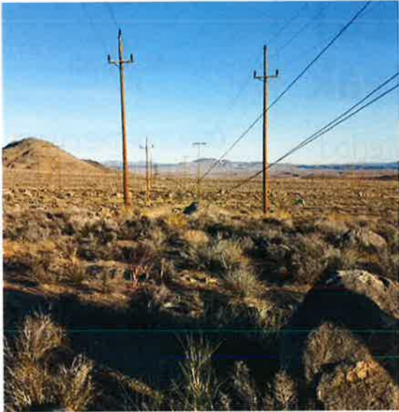
The Control-Silver Peak Project will enhance safety of SCE's sub-transmission system in portions of Inyo and Mono counties.
