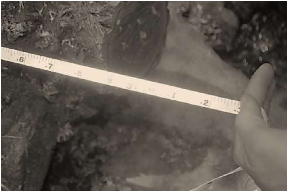
Northern corner of the structure to Rock Creek stream bank measurement of 31' 3".
