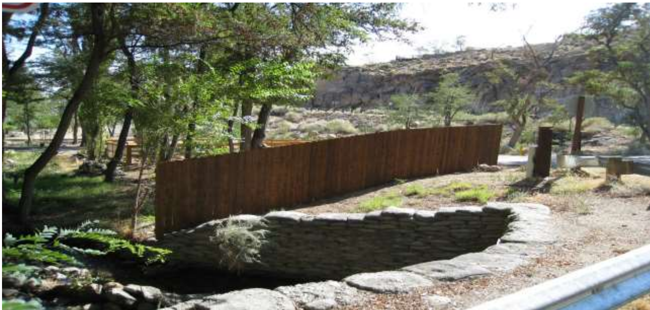
Southern view of Lot 6 prior to construction of subject structure; display of culvert intake on lower left.
